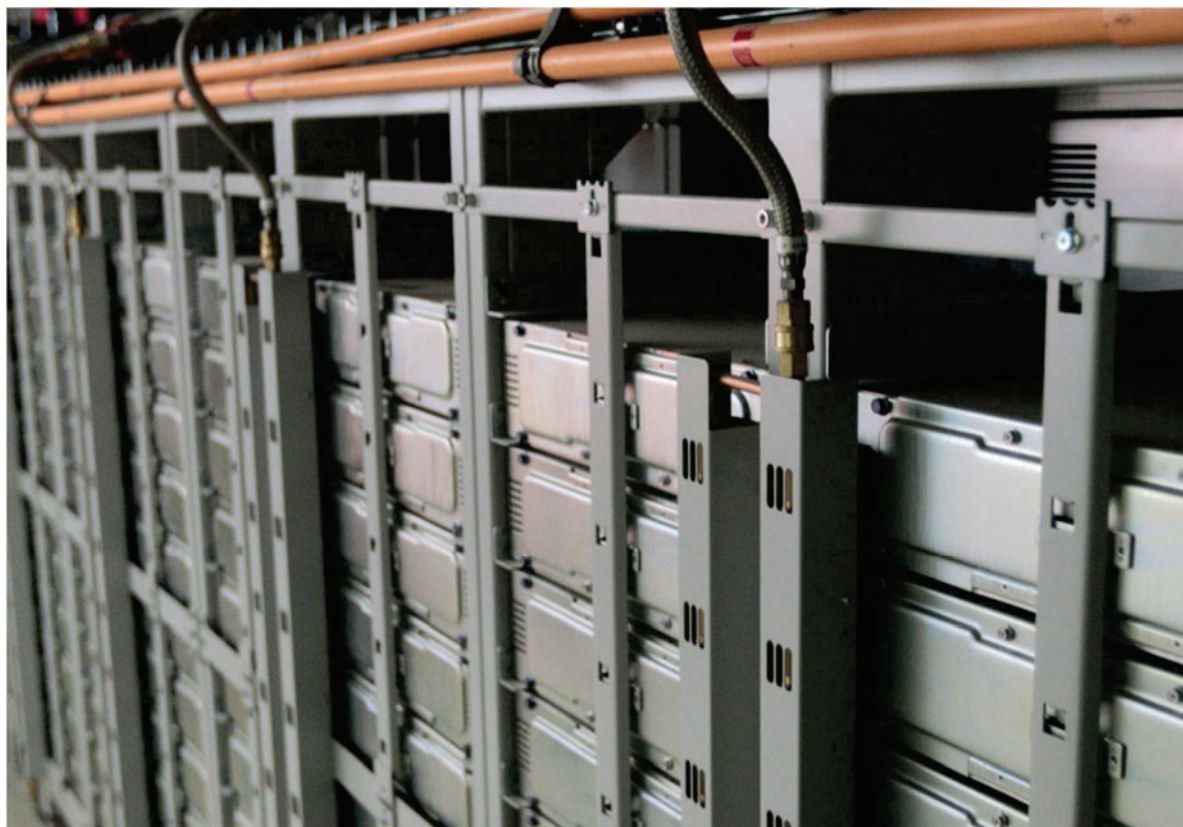
1 Figure 2: Backside of Indoor Battery Packs at Moss Landing BESS 3
